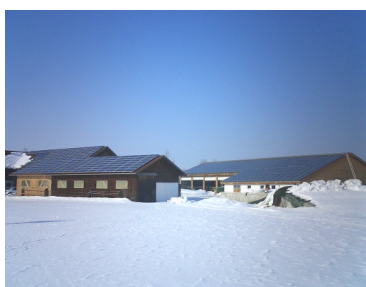
Sun-Earth brand solar modules installed at mountain with altitude more than
